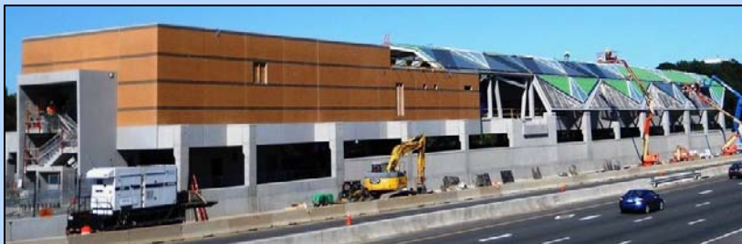
VISION OF THE FUTURE: Construction is past the 70 percent mark at the Wiehle Avenue Metrorail Station at the end of Phase 1. This station is the prototype for all Phase 2 stations except for the station at Dulles Airport.
