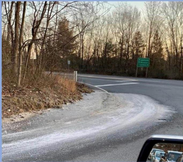
Drainage Issues at the Intersection of Hirst Road and 287
