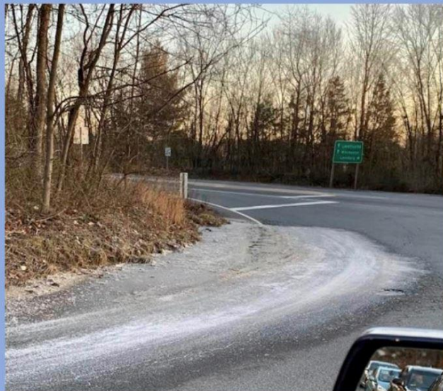
Drainage Issues at the Intersection of Hirst Road and 287
